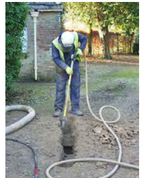
Root investigations using Airspade for an Impact Assessment as required by LPA
